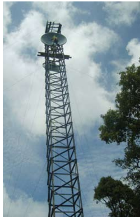
Installation technician adjusts one of the two repeater antennas.
